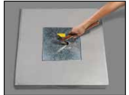
6-After screeding has cured, use hammer to knock and loosen the disposable lid before hooking it out.
